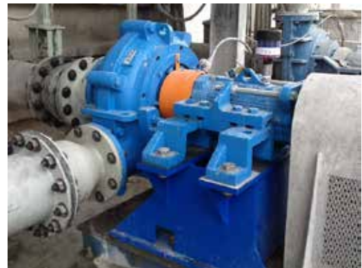
Ball mill discharge in Phosphate plant
